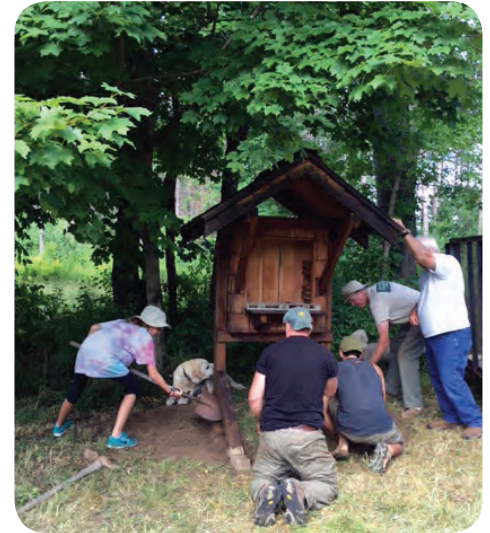
(left to right) Drew Walker, Matthew Carney, Liam Carney, Ed Robertson and Dick Edgar work to install a new trail kiosk at the Baker Woods Preserve.
